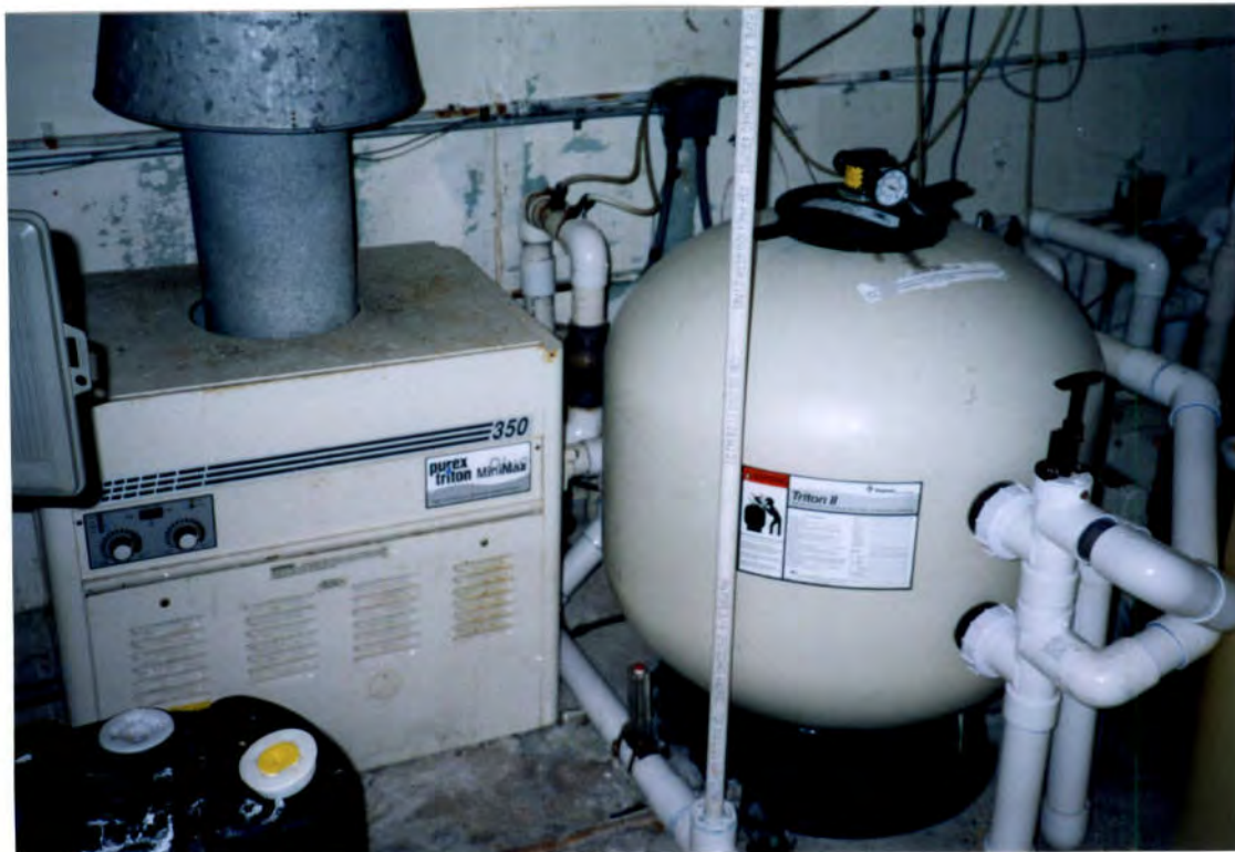
POOL AREA: Pool Equipment
