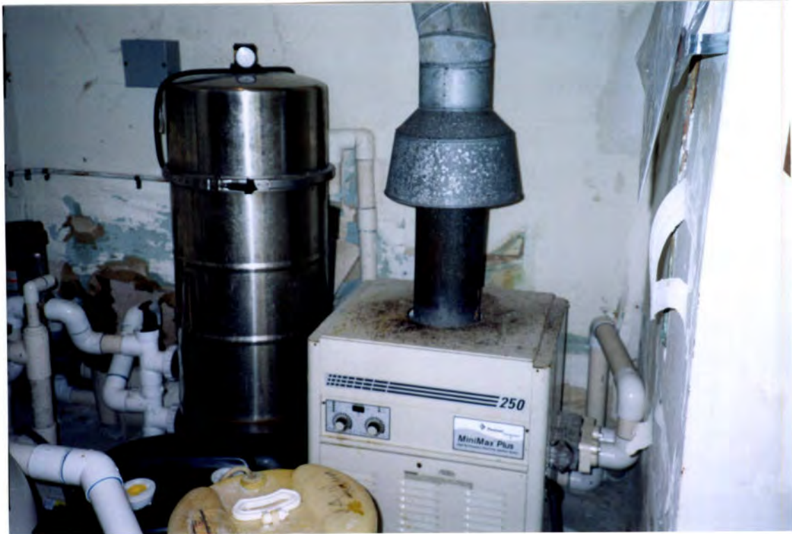
POOL AREA: Spa Equipment
