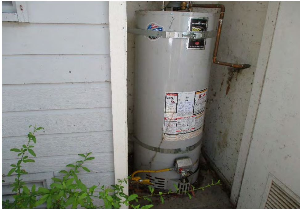
CABANA: Water Heater
