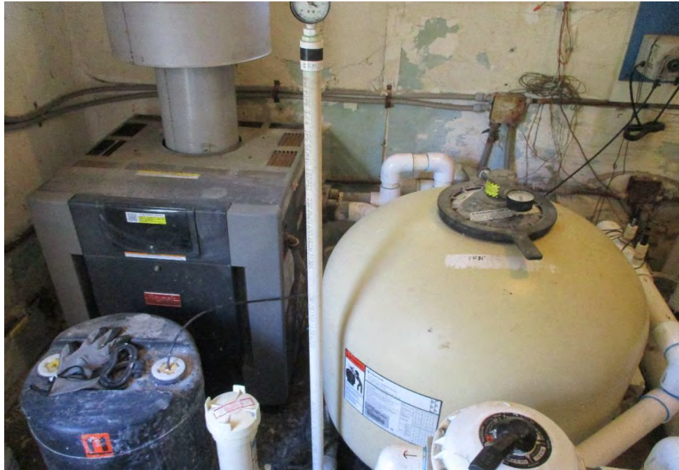
POOL AREA: Pool Heater / Filter
