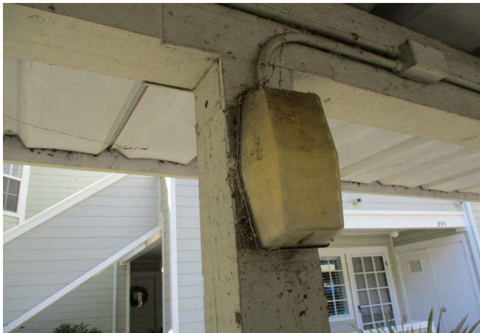
LIGHTING: Carport Lights
