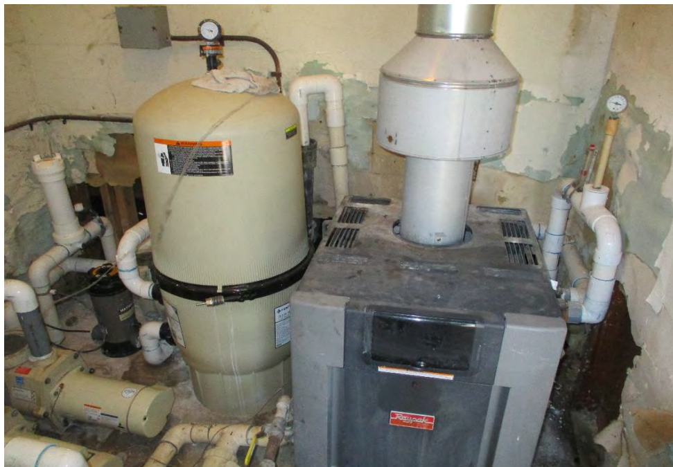
POOL AREA: Spa Heater / Filter
