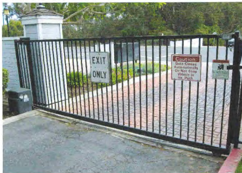
PRIVACY/FENCING: Vehicle Roll Gates / Gate Operators
